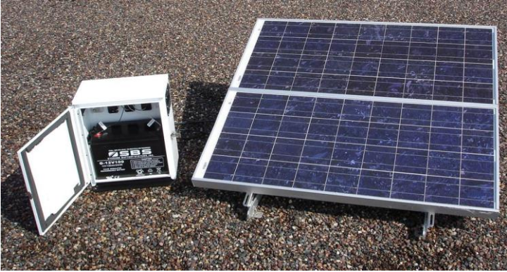
Figure 16: Solar power system (854060)
